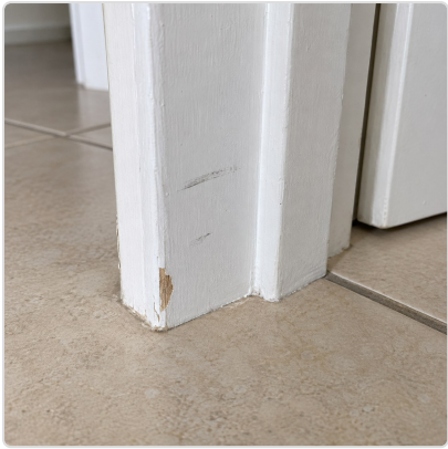
Entrance / Hall - Front door / frame 10/09/2026, 8:00:00 am AI-generated illustration conditionhq.app/samples/photos/door-frame.jpg
